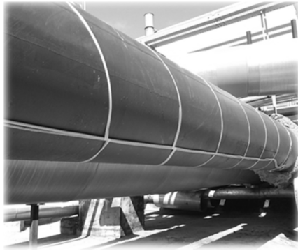
Fig. 1. Pipeline of diameter d = 400 mm and length l = 40 m heated by two linear inductors laid along the pipe
